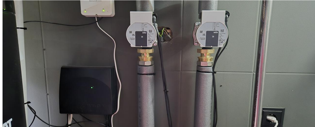
All-electric: WeHeat Blackbird, 8 kW
